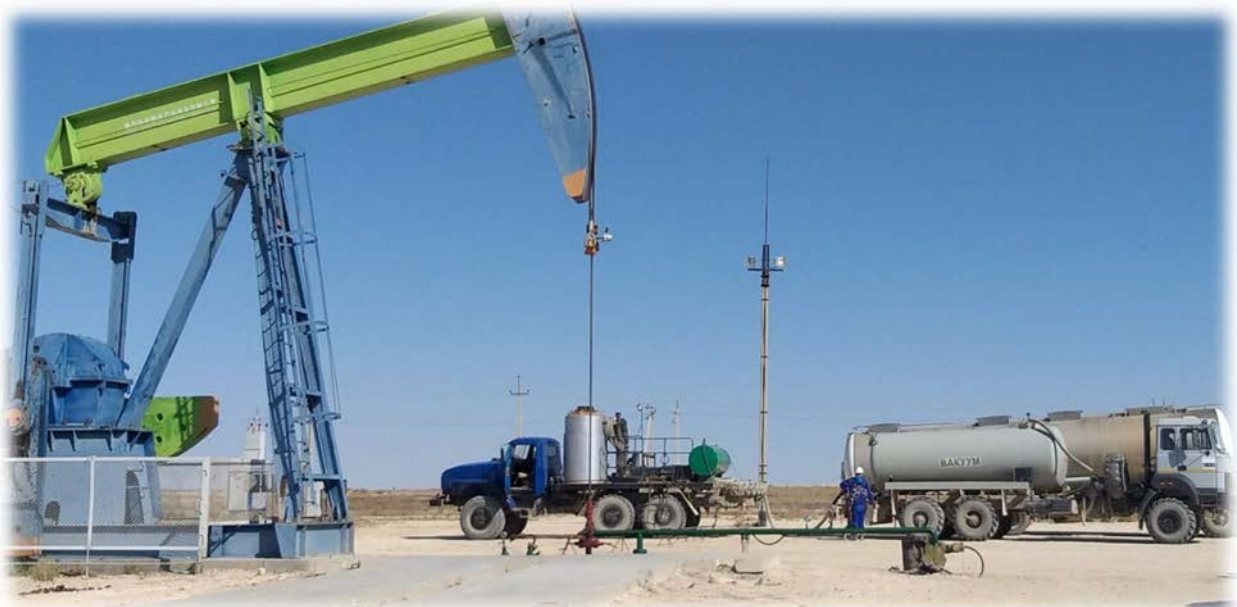
Fig.7.1. Hot Oil Unit pumps PTO from the vacuum truck into the wellhead annulus
