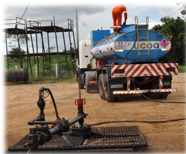
Fig.6.1. Hot Oil Unit connected to the wellhead annulus via high pressure hose
